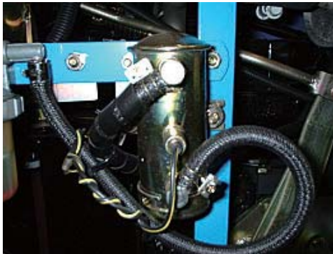
B. Fuel pump Fuel supply electromagnetic pump + Secondary fuel filter
